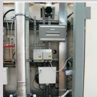
Typical service void - Electronic Control
