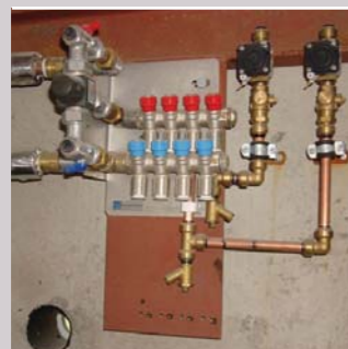
Single TMV Manifold provide water control to two cells
