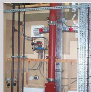
Typical service void - Pneumatic Control
